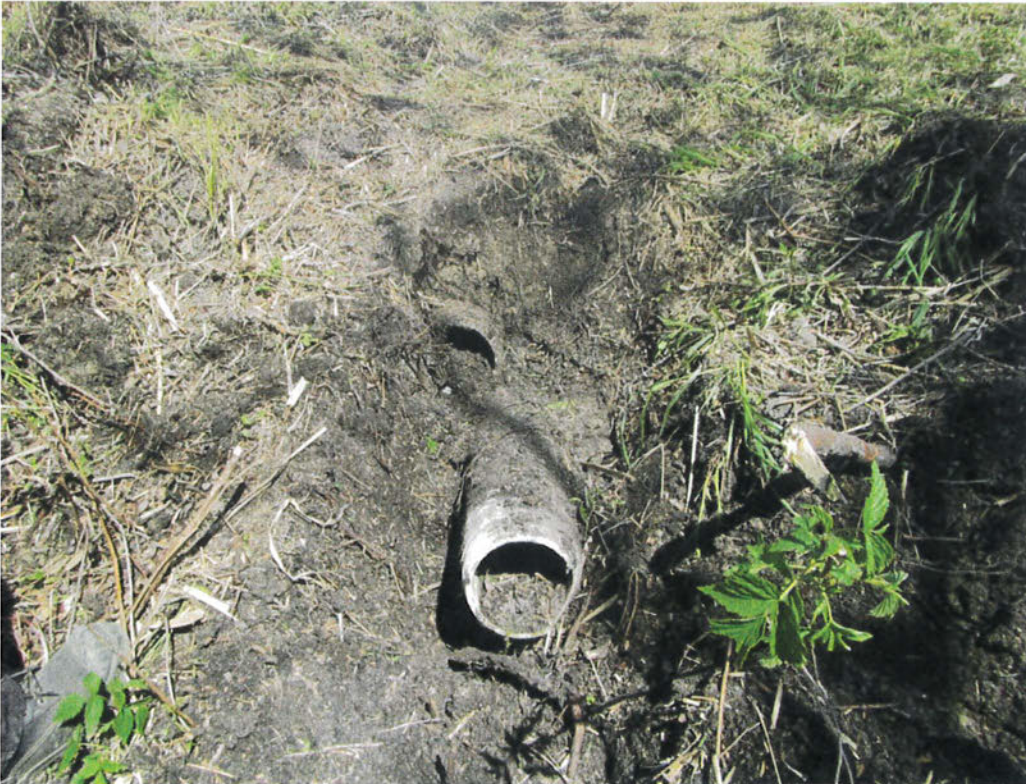
Photo 2: Abandoned discharge pipes on outer slope
