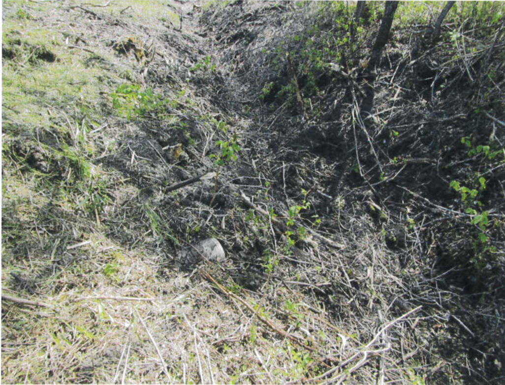
Photo 1: Abandoned discharge pipe on outer slope
