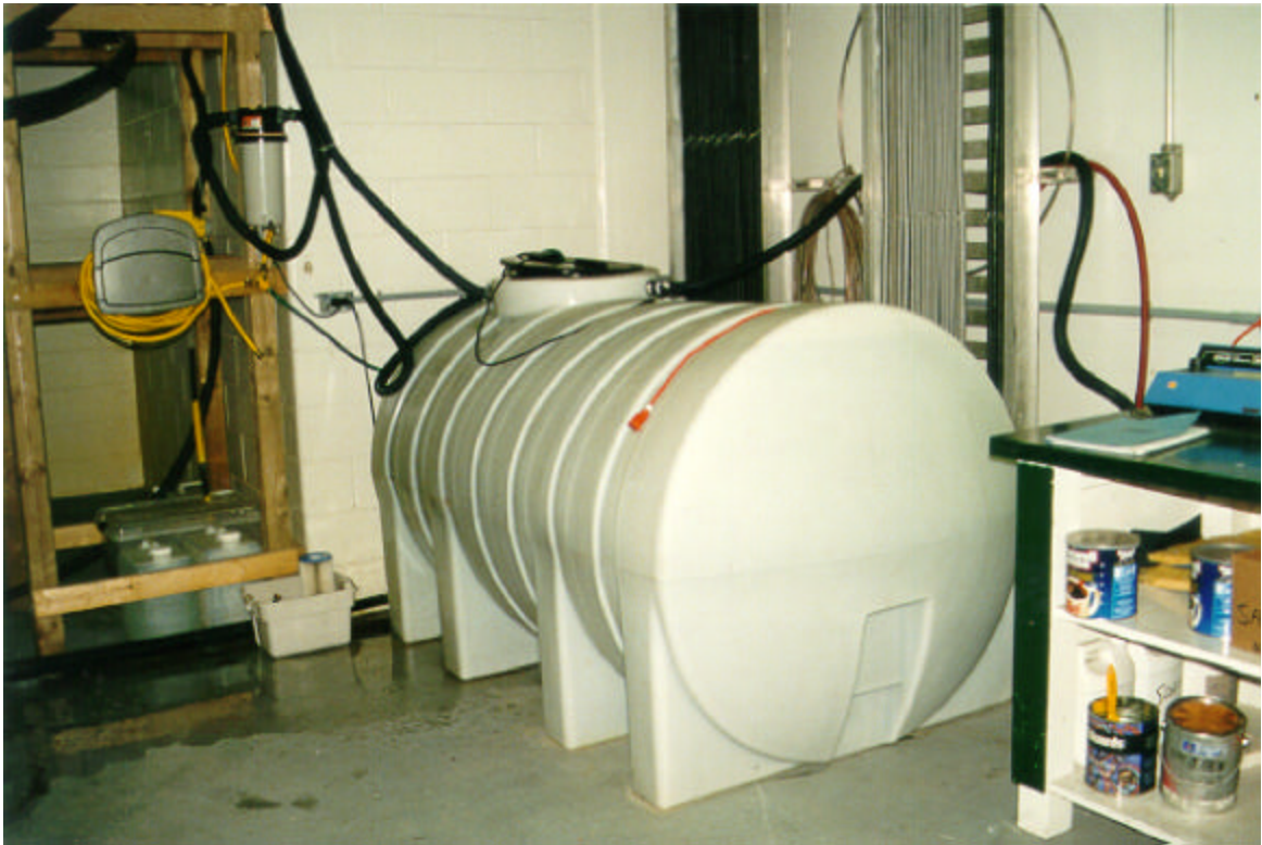
River water holding tank Figure 3-6
