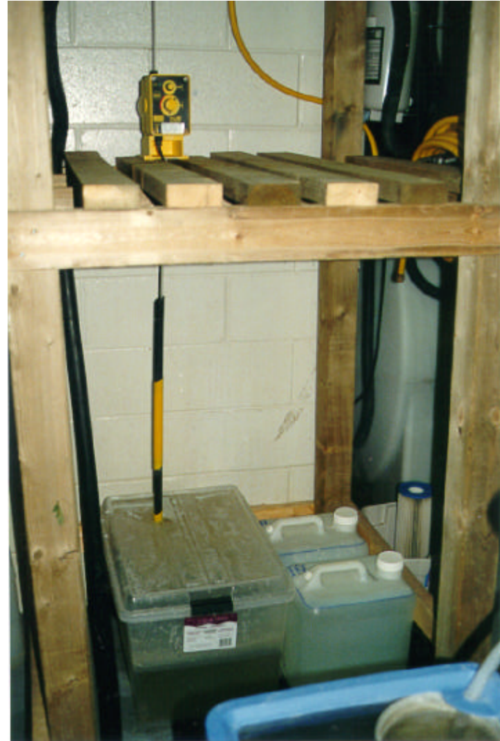
Ammonia NH 4 Cl stock container and dosing pump Figure 3-13
