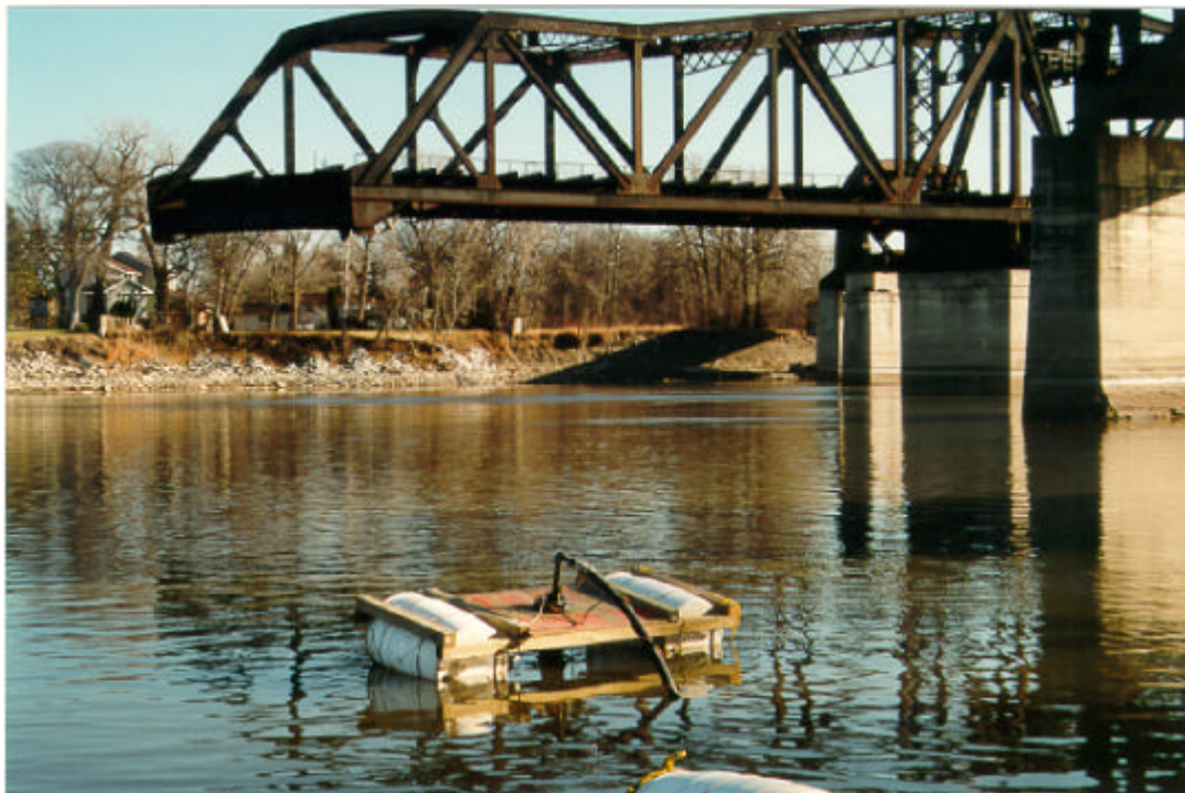
River water supply pump located on the Red River adjacent to the Bergen Cut-Off
