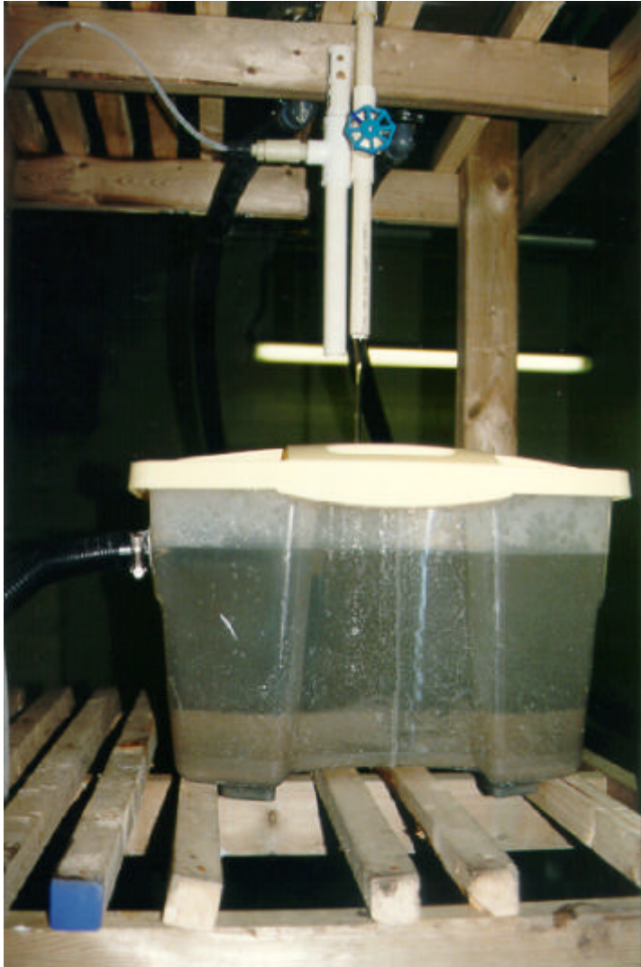
Ammonia mixing chamber on water tower Figure 3-12
