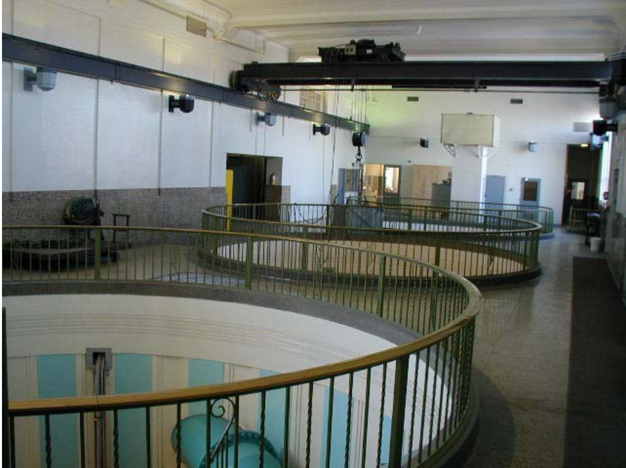
Figure 2.3 -Main Building Looking South – View of 3 Pump Wells
