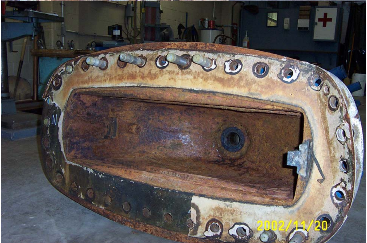
Fig. 5.1 View of Valve Body (top) and Bonnet (bottom). Note missing guide on North side.
