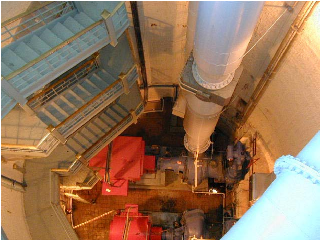
Figure 2.5 - Pump Well Number 1 - Looking Down at MP5. The suction valve is on the far right. The pump (MP5) is next to it. The motor is on the left (red).
