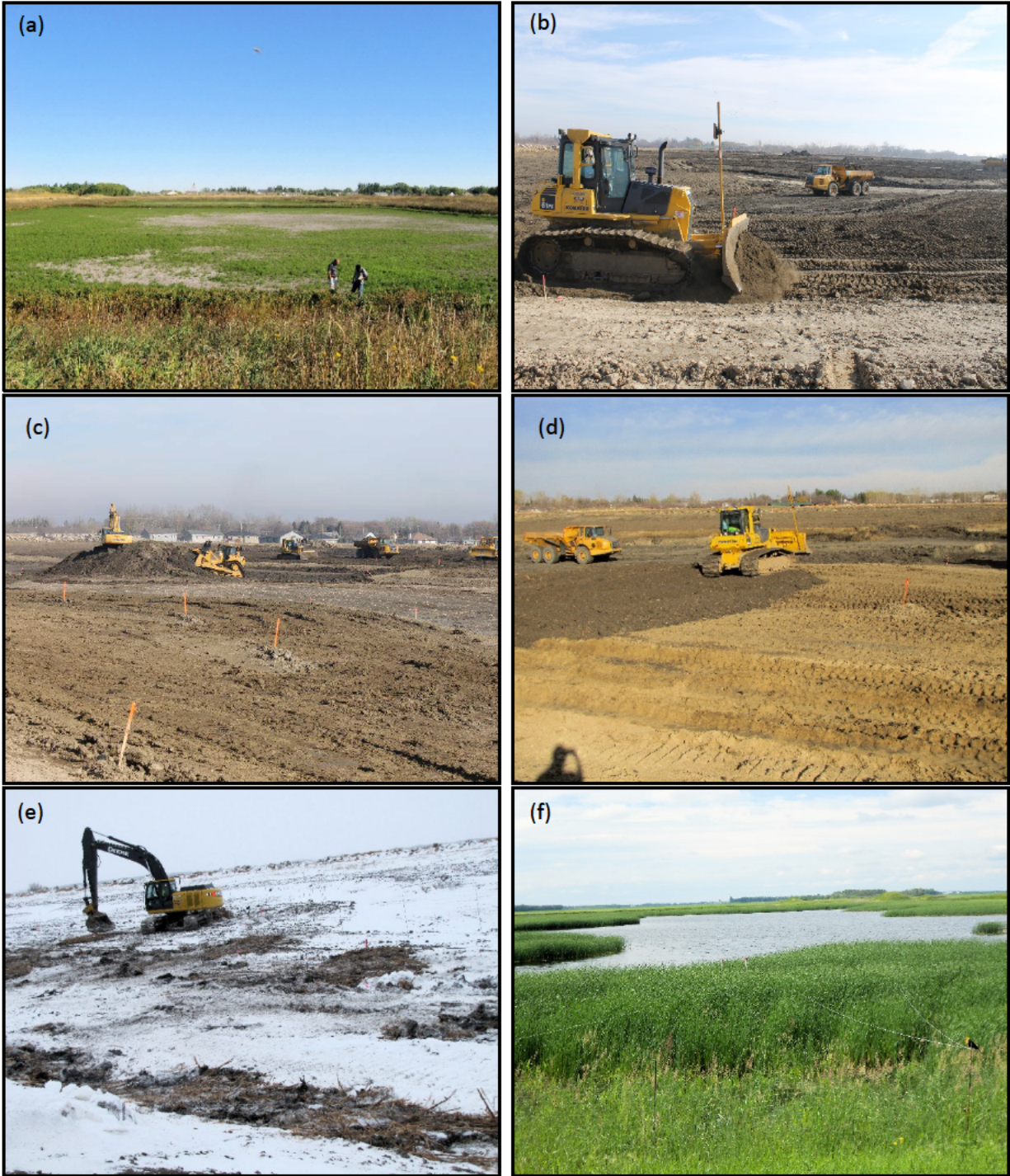
Figure 3. (a) Primary cell before construction of the wetland (September 7, 2011) (b) recontouring of the primary cell (October 16, 2012) (c) stockpiled biosolids and a constructed wetland bench (October 16, 2012) (d) spreading of biosolids on a wetland bench (October 16, 2012) (e) cattail plants placed within divots on wetland benches (November 28, 2012) (f) wetland vegetation in the second growing season (June 26, 2014).
