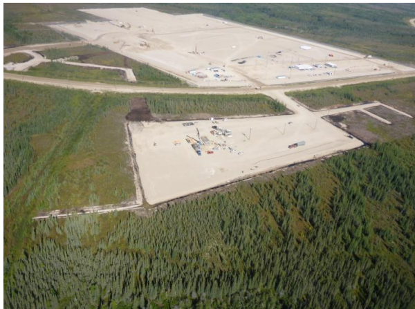
Photo 2 Aerial view of Keewatinohk Converter Station showing extent of development in August 2015
