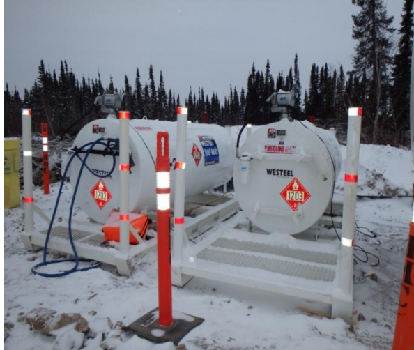
Photo 26 A spill containment system for the safe storage of gasoline
