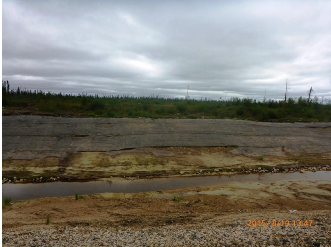
Photo 10 Damaged erosion control blanket on Keewatinohk Converter Station perimeter.
