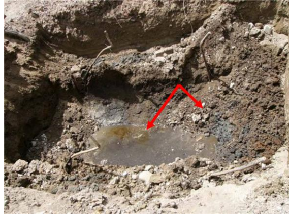
Photo 4: PHC contaminated water (note sheen on water), and soil staining
