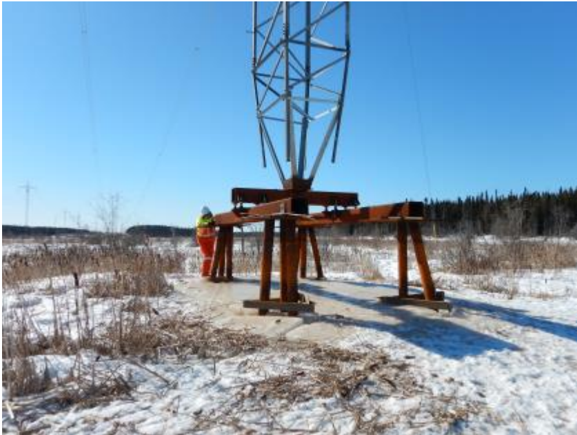
Photo 1. Photo of a transmission tower in a wetland in frozen ground conditions.
