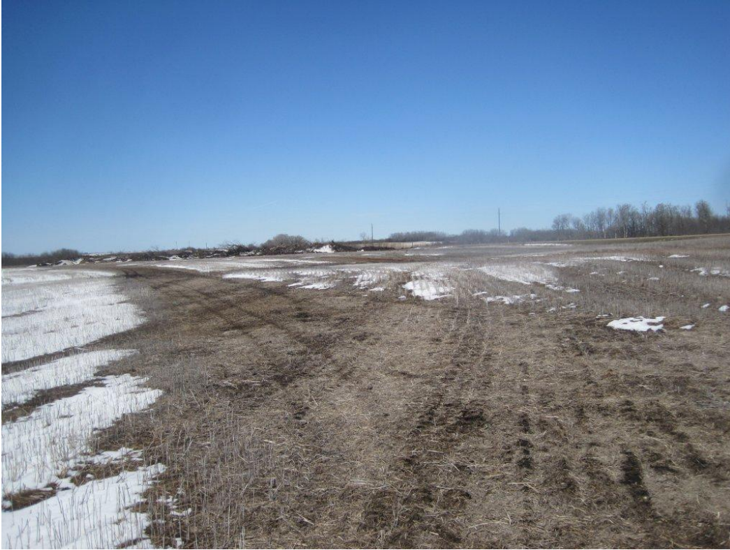
Photoplate 35 - View west at deflection point on pipeline route in NW 20-09-28 WPM.
