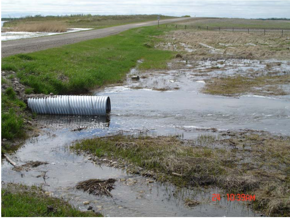
South Salt Lake - West Discharge Side - replaced 12m culvert (40 ft.) - now plastic 12m
