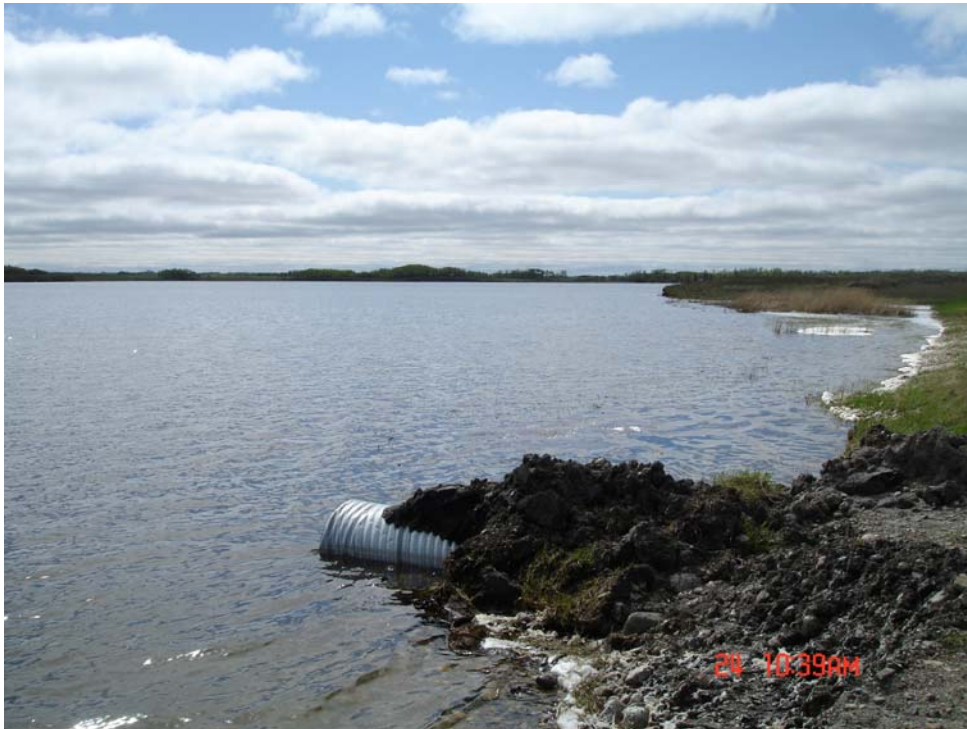
South Salt Lake - East Inlet Side - replaced metal 12m culvert (40 ft.) - now plastic 12m
