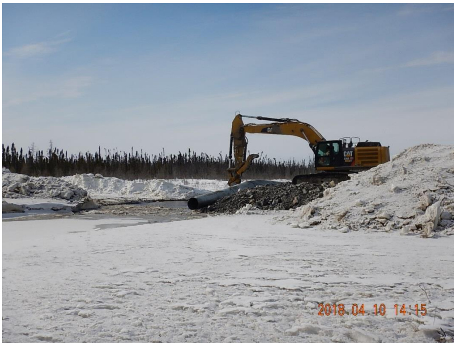
Photo 2. Removal of temporary creek crossing on winter road to Ellis Esker, April 10, 2018
