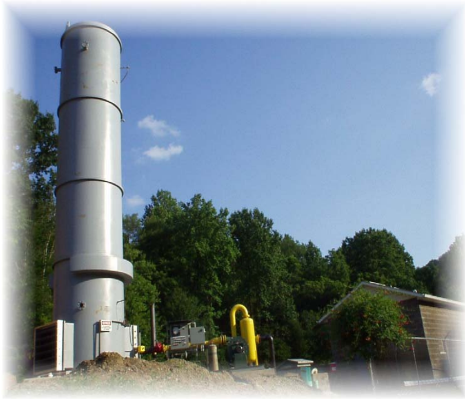
Photo 9: Typical Landfill-Gas Recovery System
