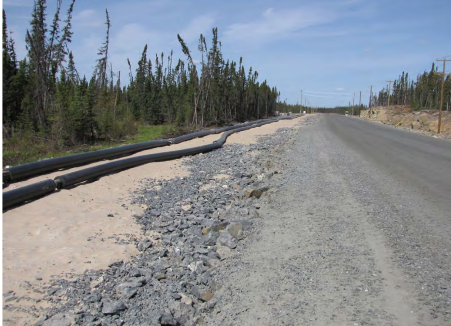
Photo 3 - Corridor of the Pipeline System (along the Lalor Access Road from Lalor site to PR 395).
