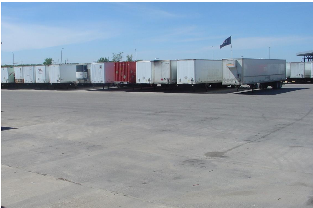
Figure 2: Trailer holding area. Note concrete surface, evidence of staining.
