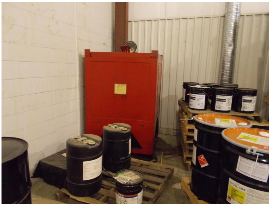
PHOTOGRAPH 8: Showing the used oil storage tank located in the hazardous room.
