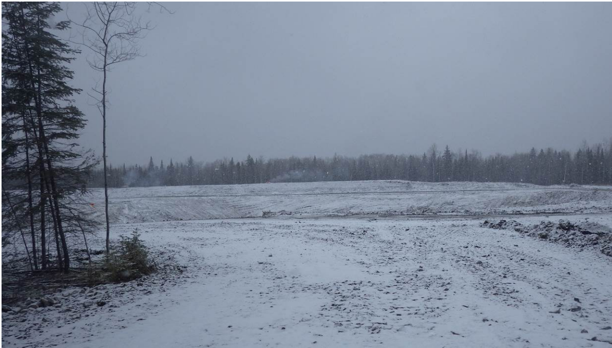
Photo 1 – Looking north along the access road at the remnant clay borrow excavation.
