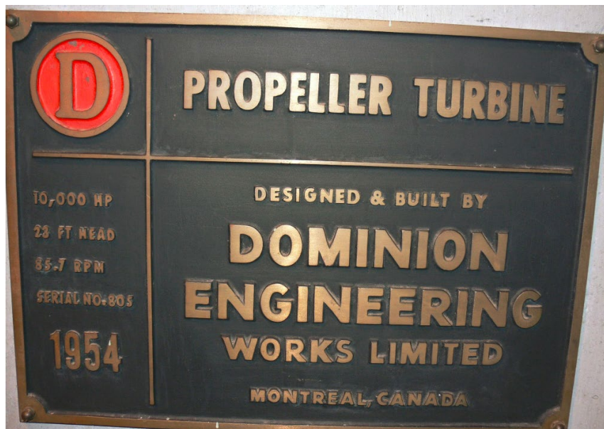
Figure 8 Unit No. 2 Nameplate Original
